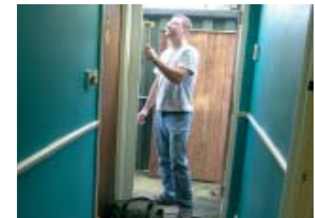
If in doubt- give it a clout. Recent new member Steve Hall works on the back door frame.
